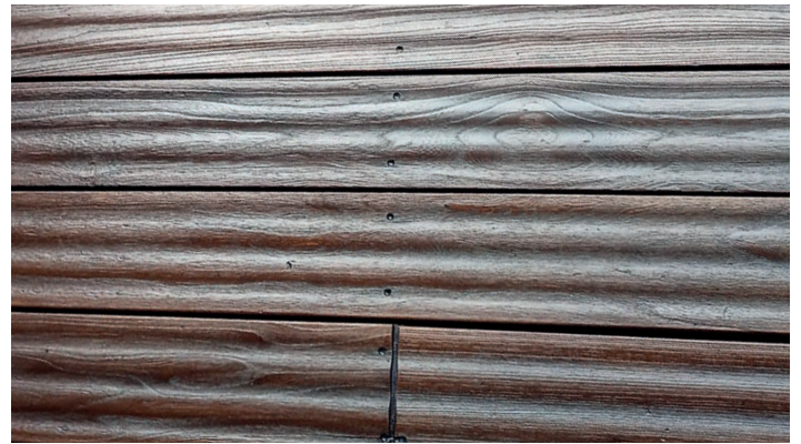
Renovated deck made from thermally treated ash after finishing with DeckFinish Color in dark brown.
